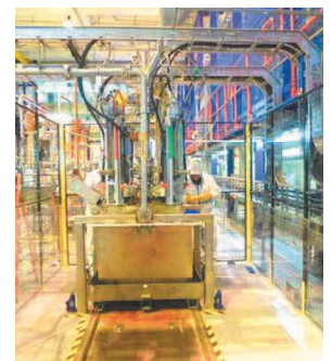
The GeoMelt® rig as installed in the NNL Central Lab.
